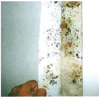
Moisture can accumulate behind vinyl wallcoverings.
