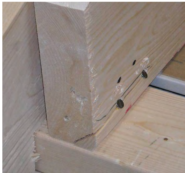
Figure 10 – Splitting of ceiling joist during installation of toe-nails
