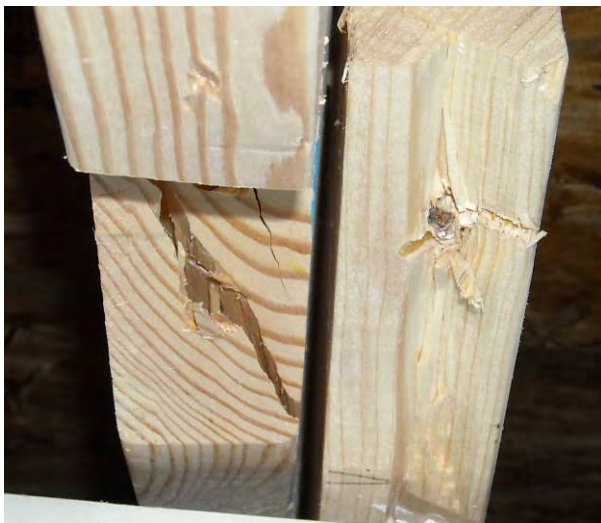
Figure 17 – Pull-through failure of all ring-shank nails
