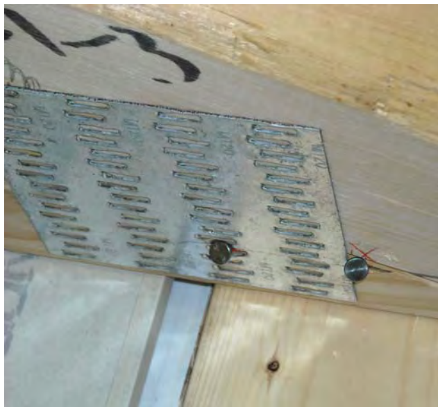
Figure 19 – Installation of one nail through the truss plate and one nail adjacent to the truss plate
