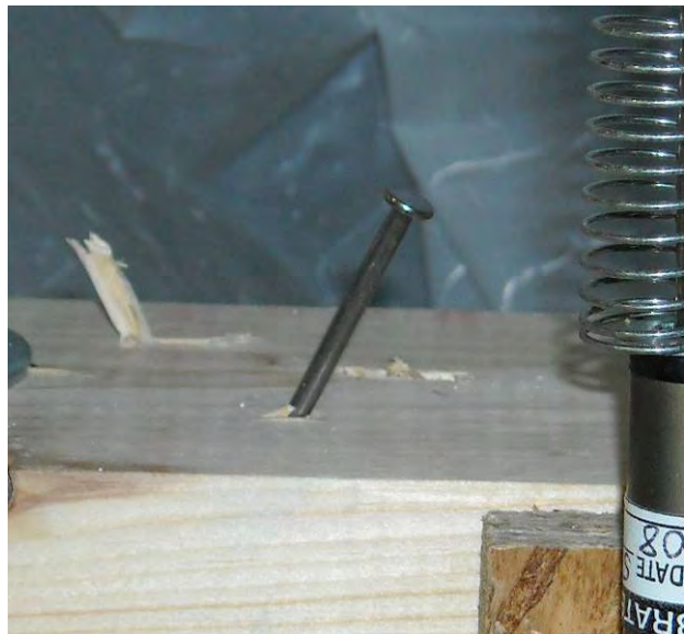
Figure 13 – Nail after pulling through rafter
