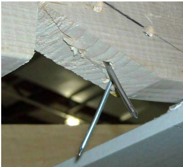
Figure 12 – Nail withdrawal and rafter splitting
