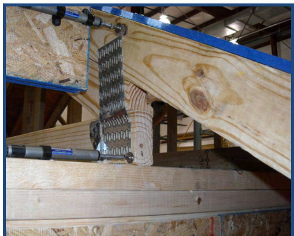
Figure 14 – Truss member displacement and metal connector plate deformation at heel joint (Specimen A)
