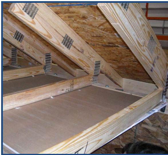
Figure 11 – Gypsum fastener tear-through (Specimen A)
