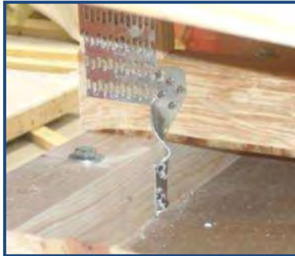
Figure 15 – Buckling of hurricane clip (Specimen C)
