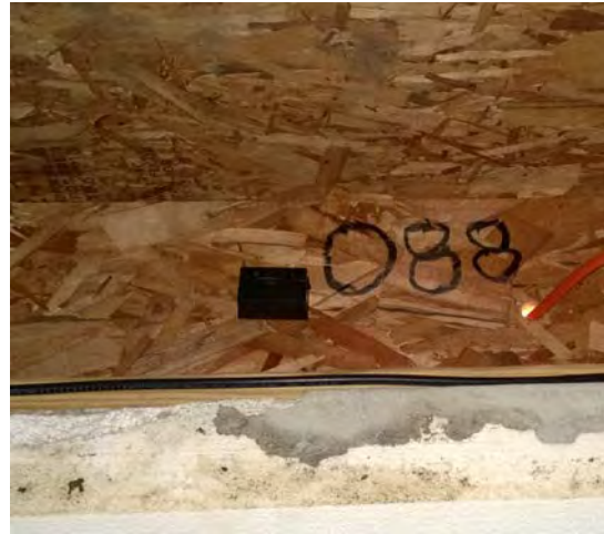
Figure 6. Sensor installed in the rim joist
