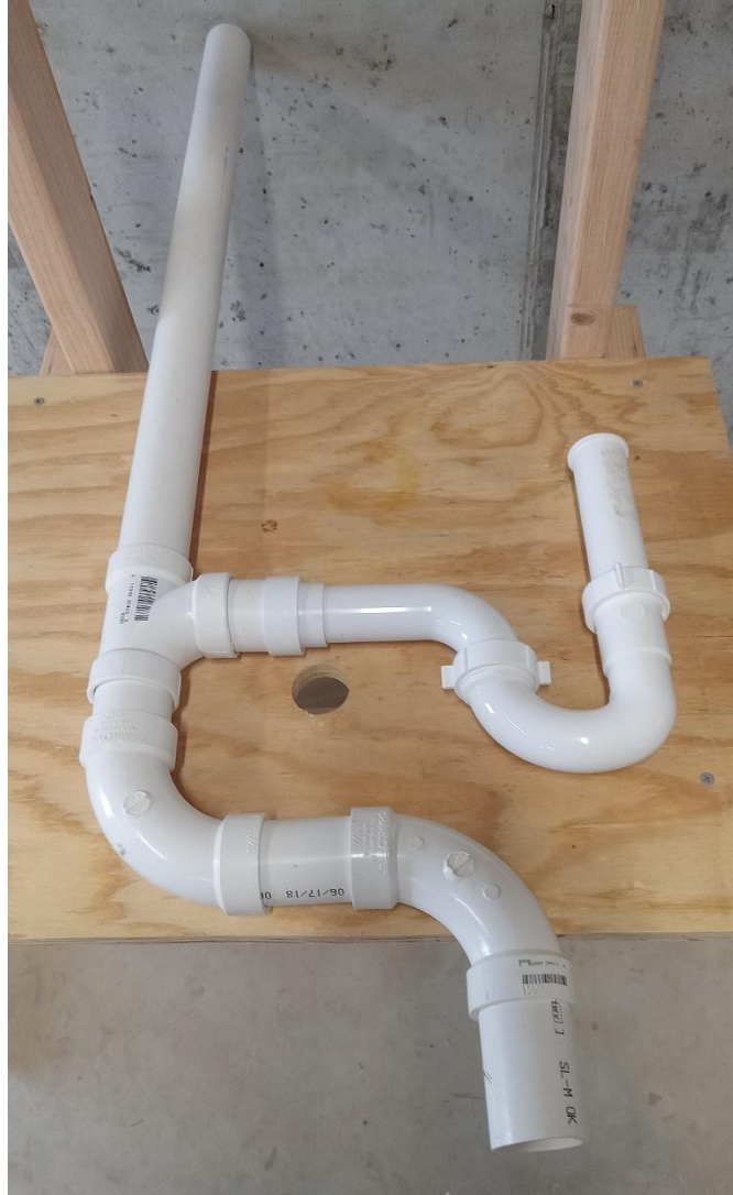
Figure 7. Complete piping assembly
