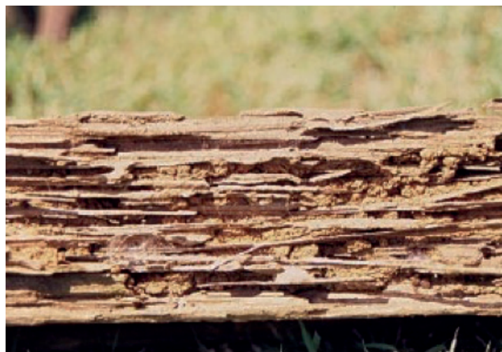
FIGURE 5. Evidence of structural termite damage
